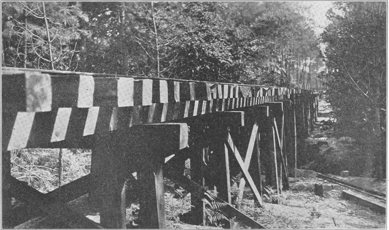
PORTIONS OF TRESTLE BUILT BY THE 20th ENGINEERS IN THE MARITIME PINE FOREST IN THE LANDES, IN SOUTHWESTERN FRANCE TO TRANSPORT FOREST PRODUCTS FROM THE WOODS TO THE MAIN LINE
